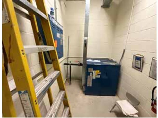
32 - ELEVATOR MACHINE ROOM
