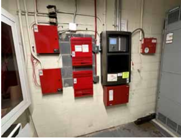
25 - FIRE ALARM PANEL
